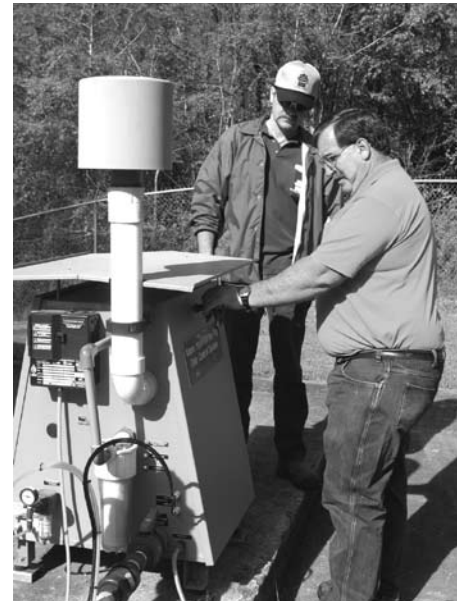
Craig Stevens and Tony Burkes opening Vapex O-Mega unit at Hot Springs Creek pump station.
