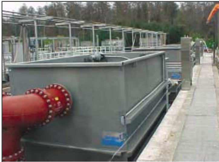
Orange County's North Plant AquaDisk® Filters.
