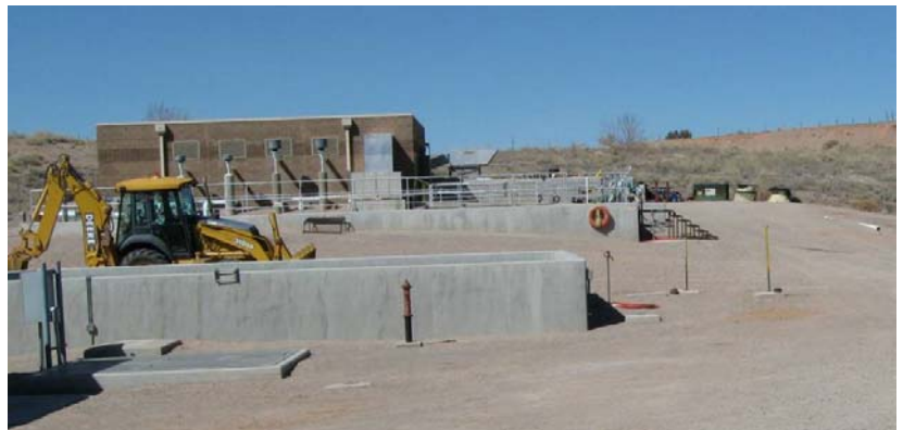
Santa Ana Water Reclamation Facility
