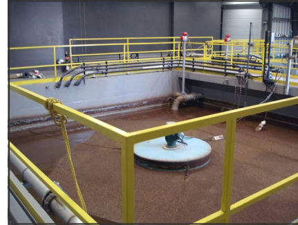
One of Quechan's batch biological reactors.
